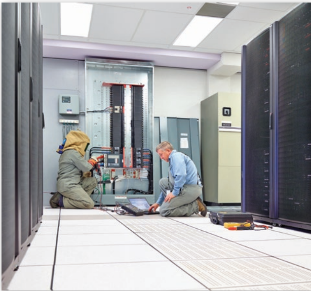
TOP: ELECTRICAL DISTRIBUTION AND CONDUIT INSTALLATION AT THE VARSONA THEATRE (DESIGN ASSIST PROJECT WITH PCL CONSTRUCTION). MIDDLE: ACTION'S SERVICE TECHNICIANS PERFORMING EXTERIOR LIGHTING MAINTENANCE AT SHELL CANADA. BOTTOM: ACTION ELECTRICAL'S TEGG TECHNICIANS COMPLETING ELECTRICAL DISTRIBUTION PREVENTATIVE MAINTENANCE SERVICES.
